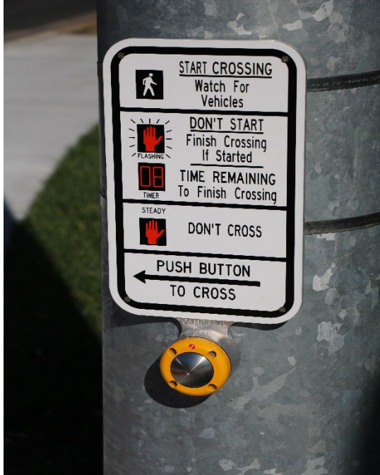
Figure 3 Traffic control signal at Canton Farm Rd. 2017.
